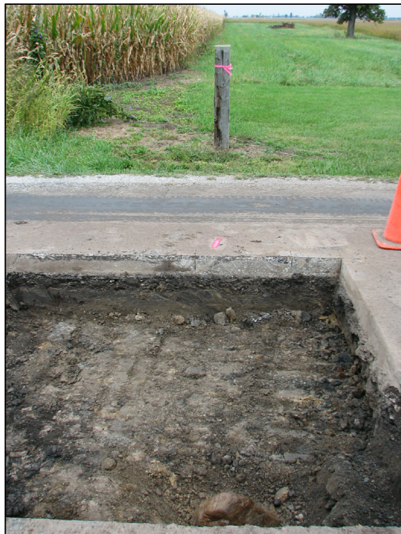
View from the south showing the found stone, and the old post on the north side of the road.
