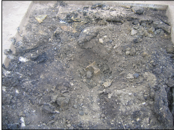
The railroad rail exposed.
