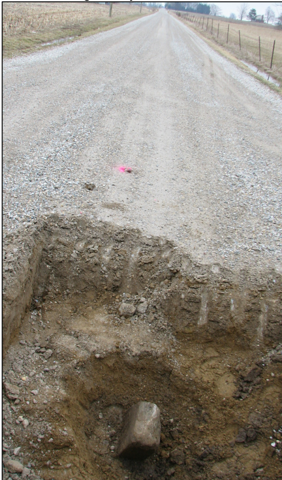
View from the west, looking across the stone and east along County Road 500 South.
