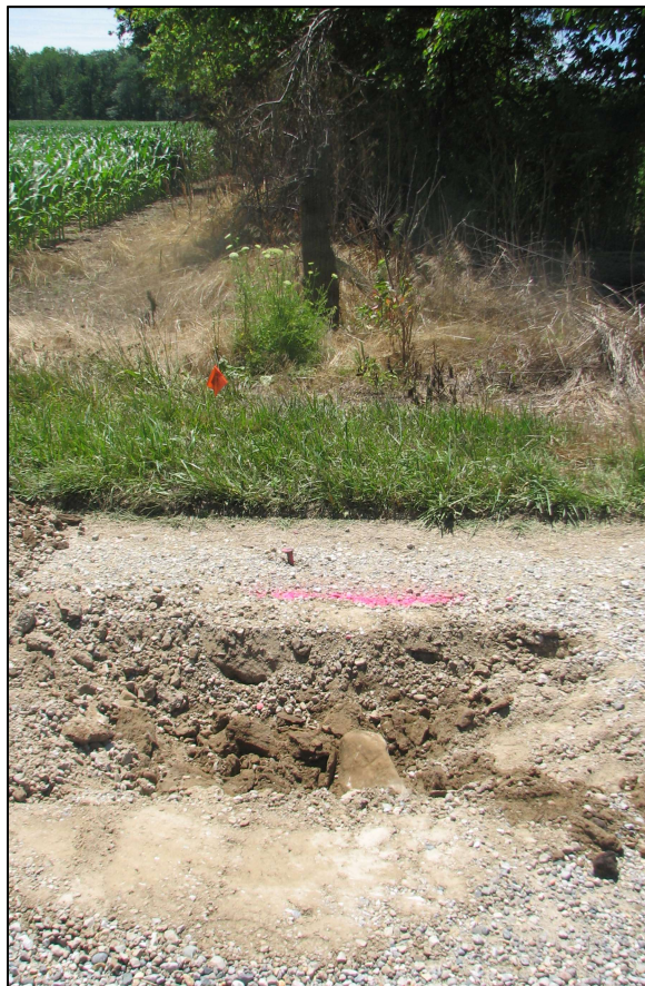
View looking across the stone to the wood end post on the south side of C.R. 700 North.
