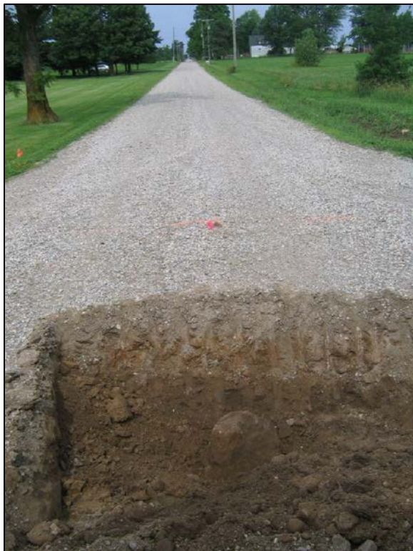
View from the east, looking across the stone and west along County Road 200 North.
