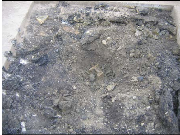
The railroad rail exposed.
