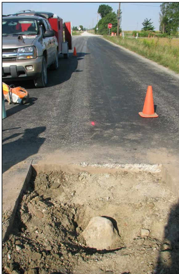
View from the east, looking across the stone and west along County Road 100 North, across U.S. 421
