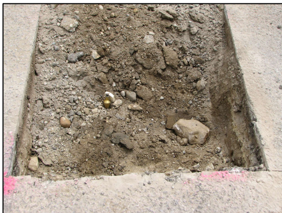
View from above and north, showing the stone and the position of the rebar as marked with a plumb-bob.
