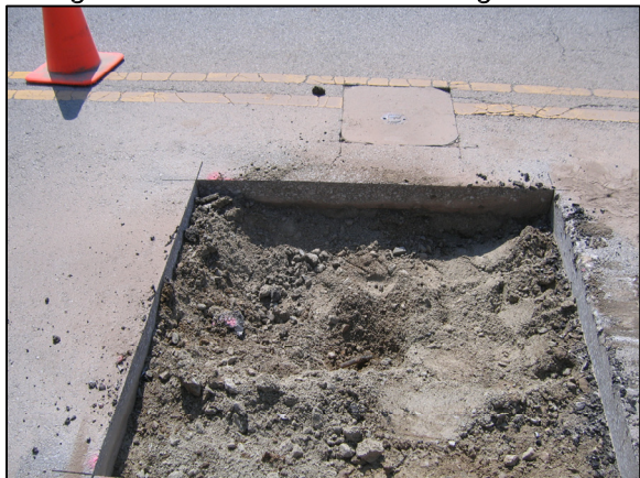
The bent rebar within the area of excavation, along with the harrison at the closing corner.
