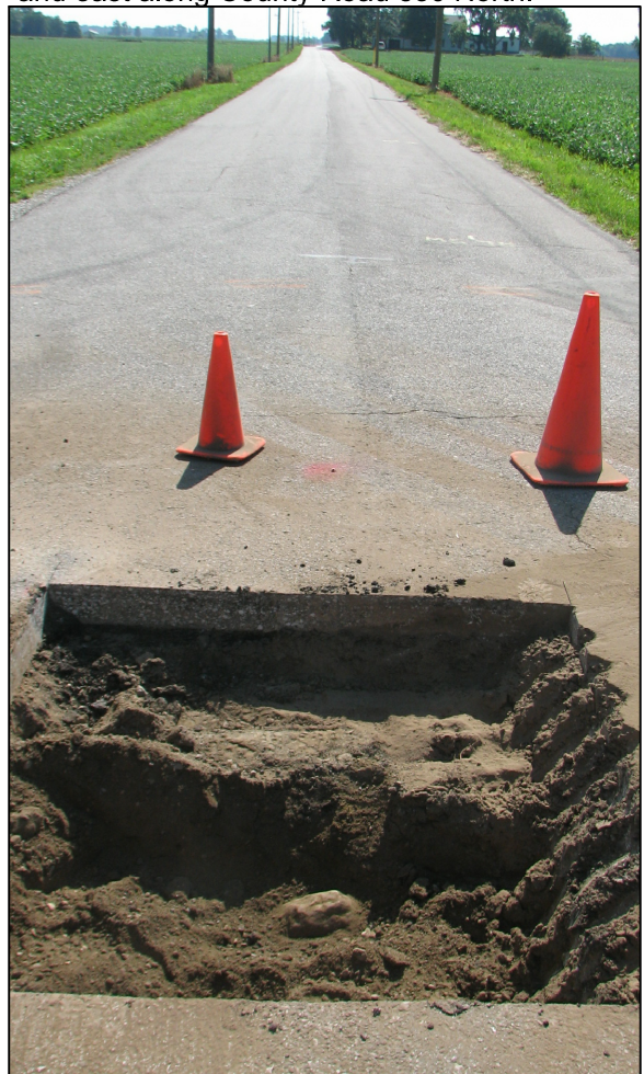
View from the west, looking across the stone and east along County Road 850 North.
