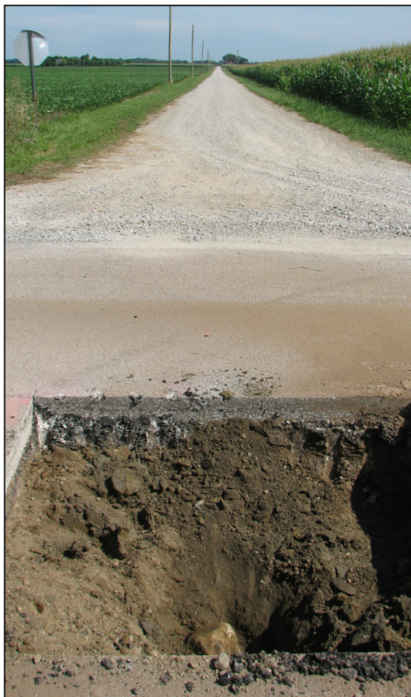
View from the south, looking across the upper stone and north along C.R. 800 East.
