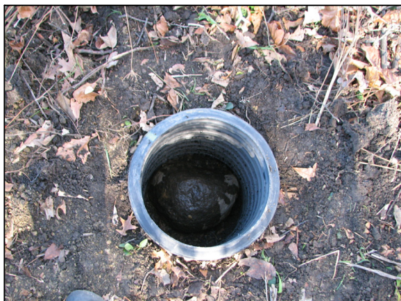
The stone within the section of HDPE storm pipe, immediately prior to being encased in concrete.
