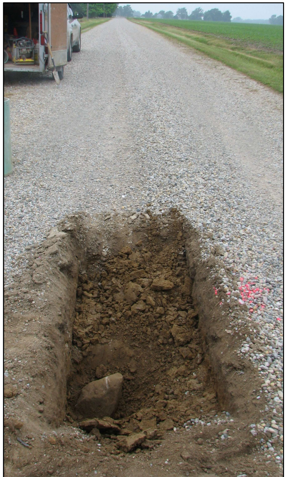
View from east, looking across the stone and west along County Road 900 North.
