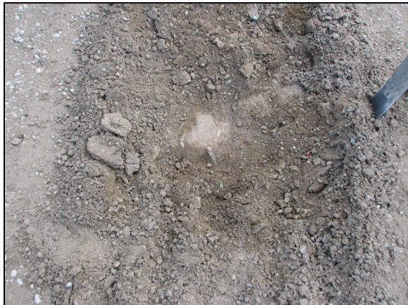
View of the stone and bent rebar from the north and above.
