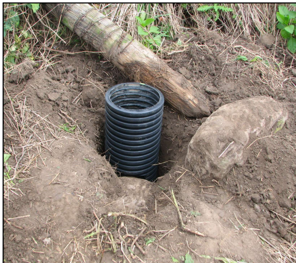
A vertical section of storm pipe, to be filled with concrete to support the Harrison monument.
