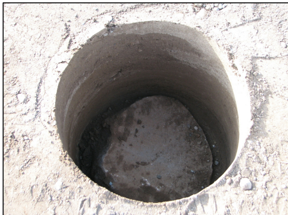
The lower stone immediately before it is encased in concrete and a harrison monument set over it.
