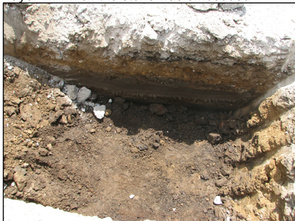
Excavation below the stone, showing the cross section of the roadway. Note the distinct clay layer in which the stone was embedded.
