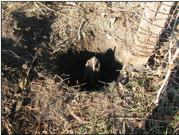
The standing post and the base of the old post, with rebar, from above and east.
