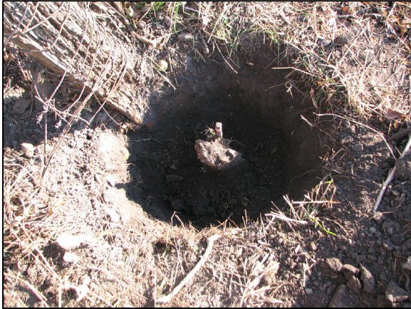
The standing post and the base of the old post, with rebar, from above.
