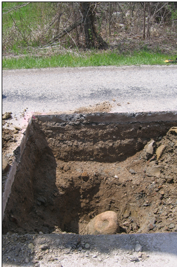
View of the stone and the wood end post on the east side of the road.
