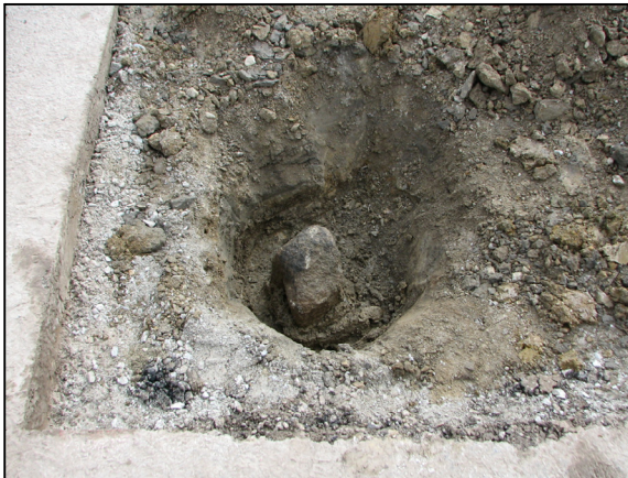
View of the stone after the rail was removed.
