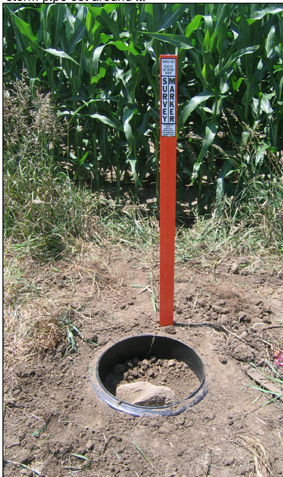
The stone with the vertical section of plastic storm pipe set around it.
