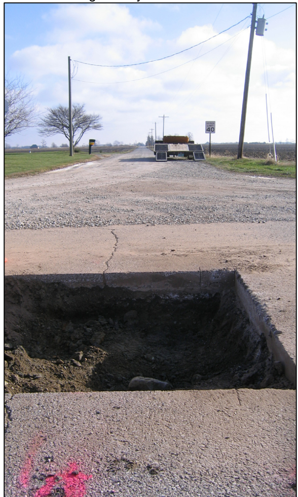
View from the west, looking across the stone and east along County Road 650 South.
