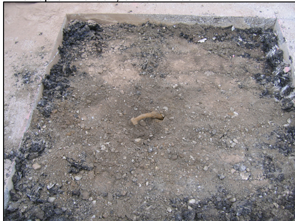
The top of the bolt, as found bent.
