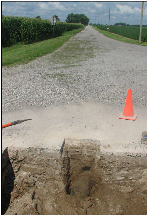
View from the west looking across the lower stone and west along County Road 50 South.
