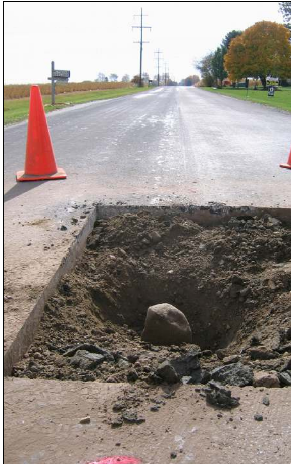
View from the north, looking across the stone and south along County Road 300 East.
