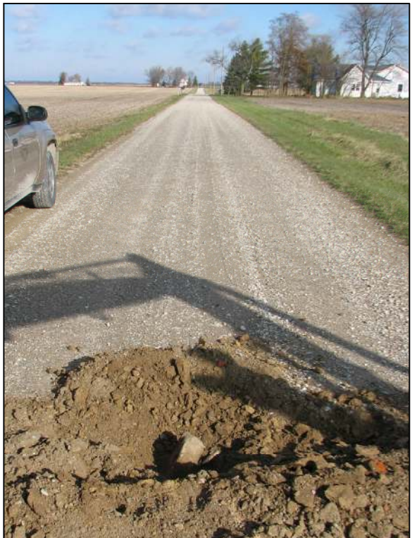
View from the south, looking across the stone and north along County Road 500 East.
