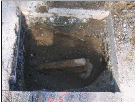
View of the rail leaning over the stone.
