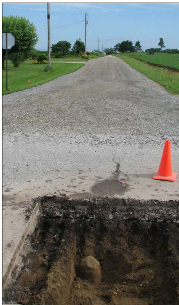
View from the south looking across the stone and north along County Road 50 South.
