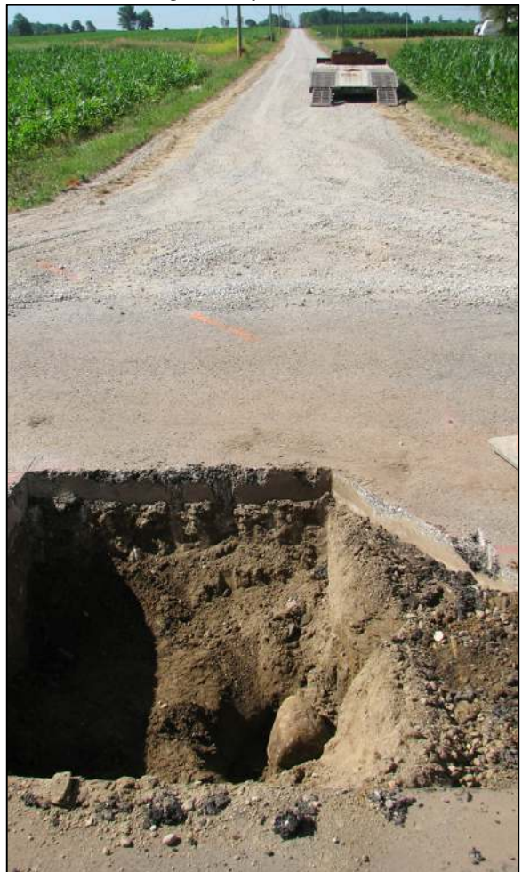
View from the north, looking across the stone and south along County Road 50 East.
