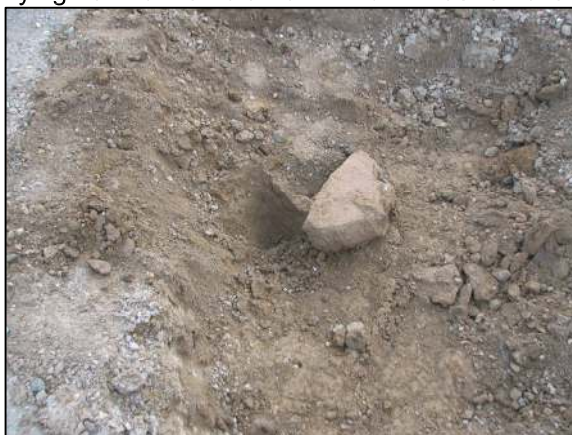
View of the stone removed from the road bed, lying next to the hole from which it was removed.
