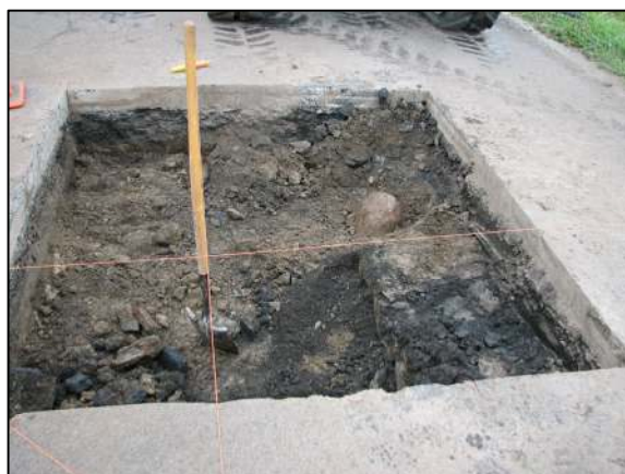
View showing the found stone and a shovel set temporarily in the position of the rail, as found.
