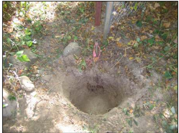
Corner 2 being excavated, showing the pipe, metal posts to the south, the in ground portion of the wood post, and a rock found on the north side of the post, presumably a brace rock.
