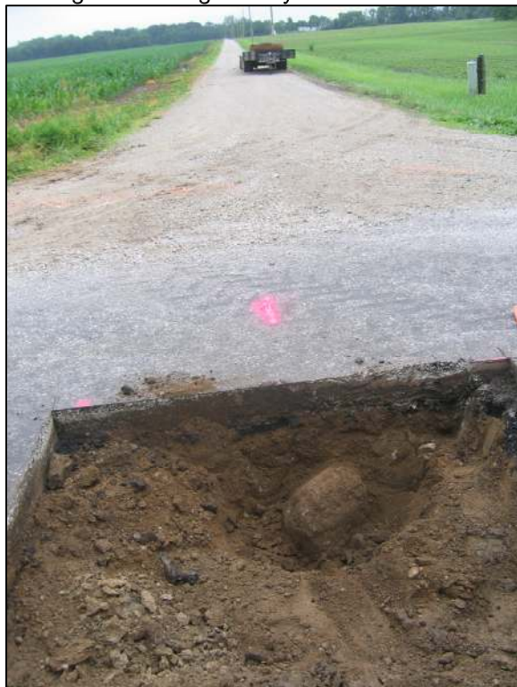
View of the top stone. View is from the south, looking north along County Road 750 East.
