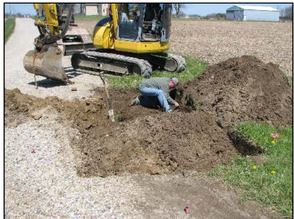
View from the south, showing the area of excavation. Brandon Miller, Miller Excavating, is inspecting the upper stone as found.
