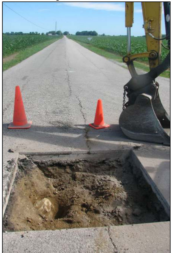
View from the south, looking across the stone and north along C.R. 1050 West.
