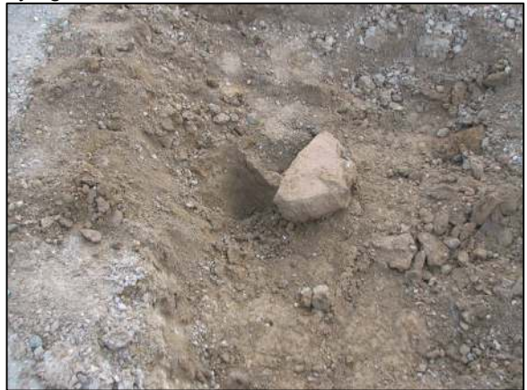
View of the stone removed from the road bed, lying next to the hole from which it was removed.
