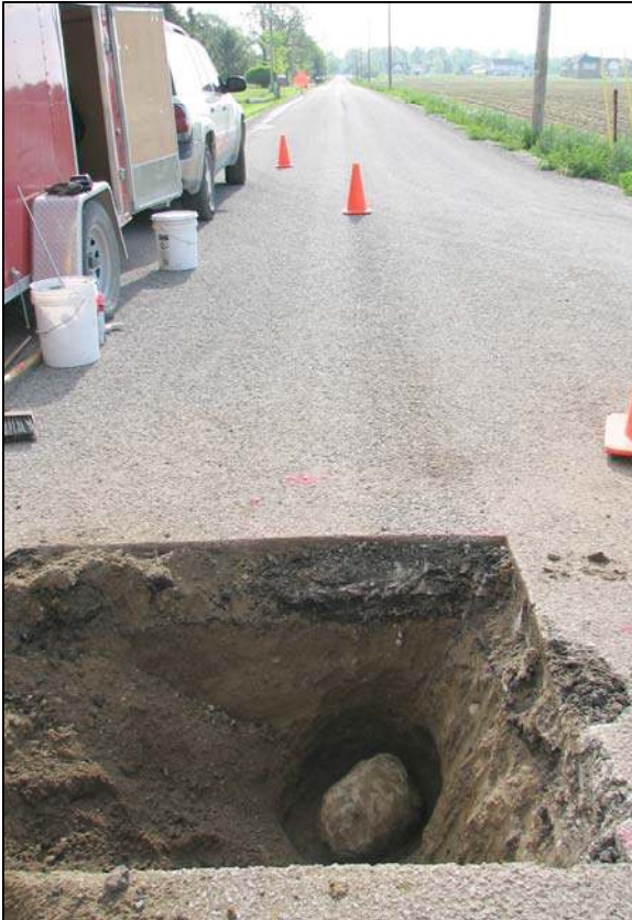
View from west, looking across corner stone and along County Road 400 South to the east.
