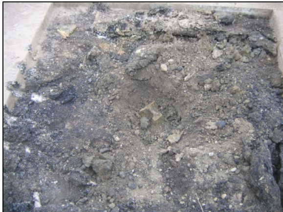
The railroad rail exposed.
