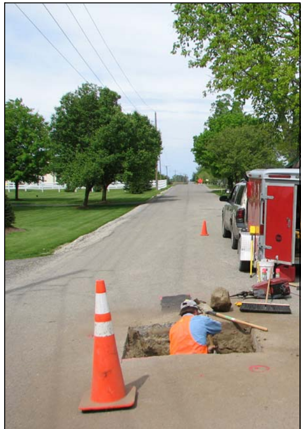
View from east, looking across hole and along County Road 400 South to the east. The upper stone is visible on the road surface.
