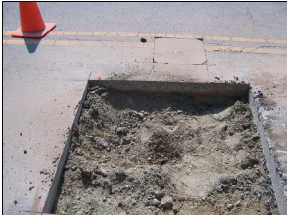
The bent rebar within the area of excavation, along with the harrison at the closing corner.
