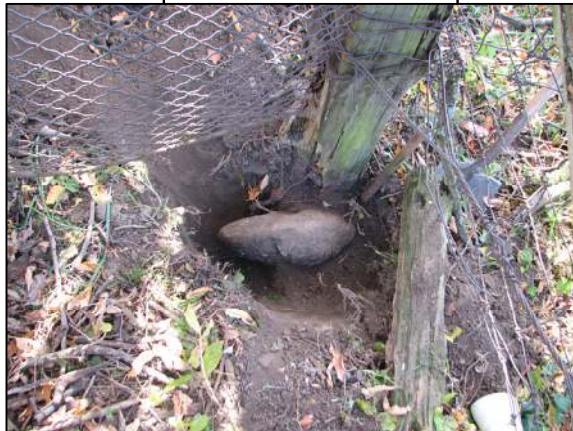
The stone exposed at the base of the post.
