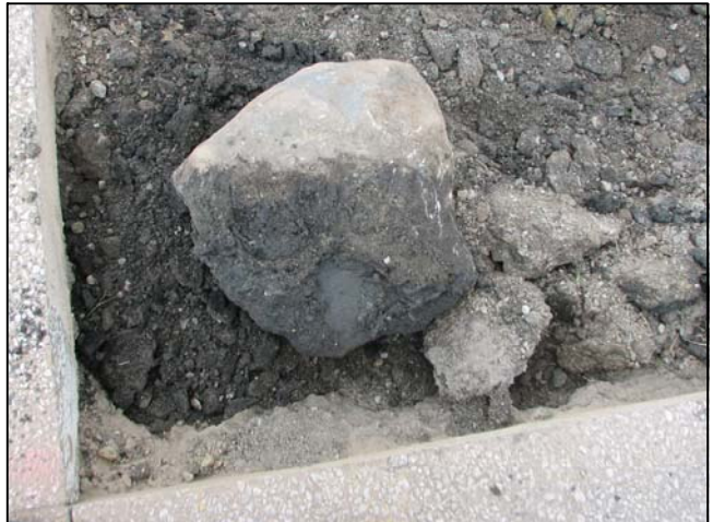
Corner stone removed from ground, showing extent to which stone was embedded in clay. Approximately 10" of stone was in clay and 7" protruding into bottom of road bed.
