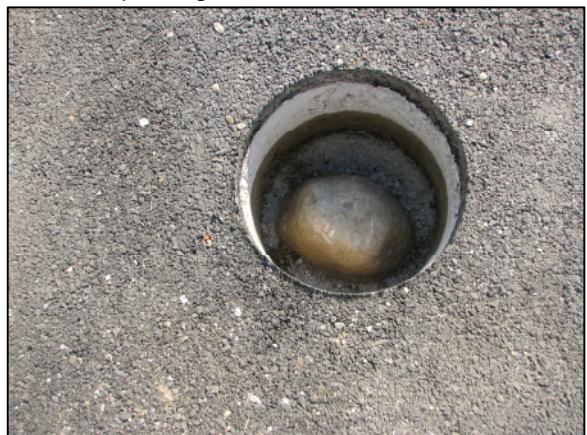
View of the stone from above, immediately prior to the top being encased in concrete.
