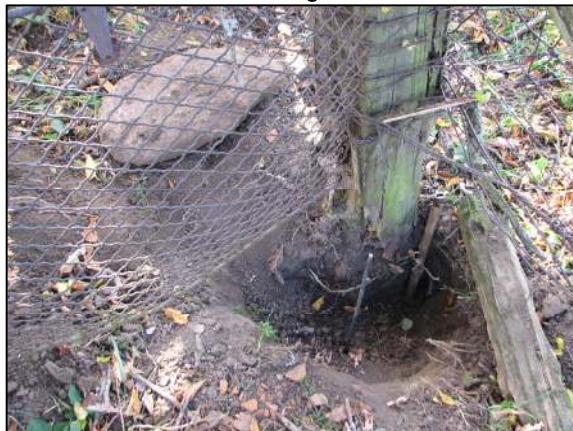
The post and iron pipe. The small rebar is in the position at which the harrison was subsequently set. The stone is on the ground to the left.
