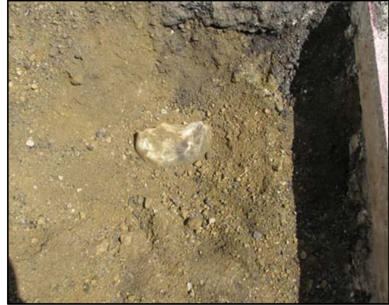
Stone against which the iron pipe was situated. Stone is in road sub-base, not clay.
