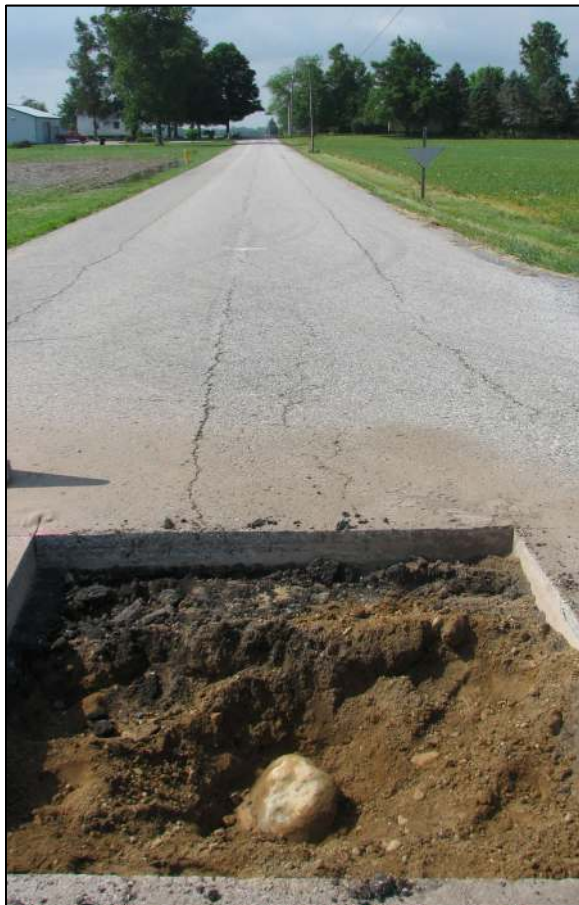
View from north, looking across the stone and south along County Road 1050 West.
