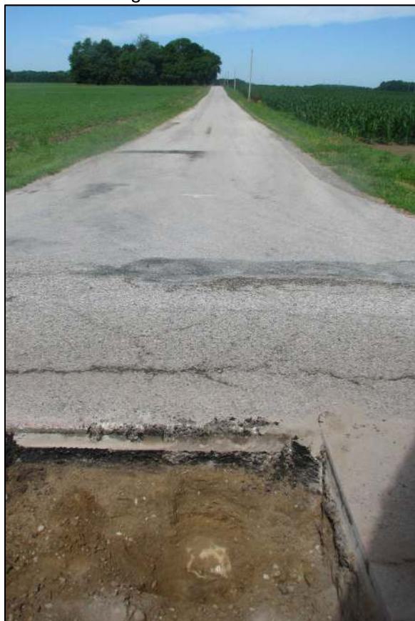
View from the east, looking across the stone and west along C.R. 800 North.
