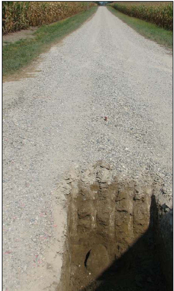
View from the south, looking across the stone and north along County Road 800 East.
