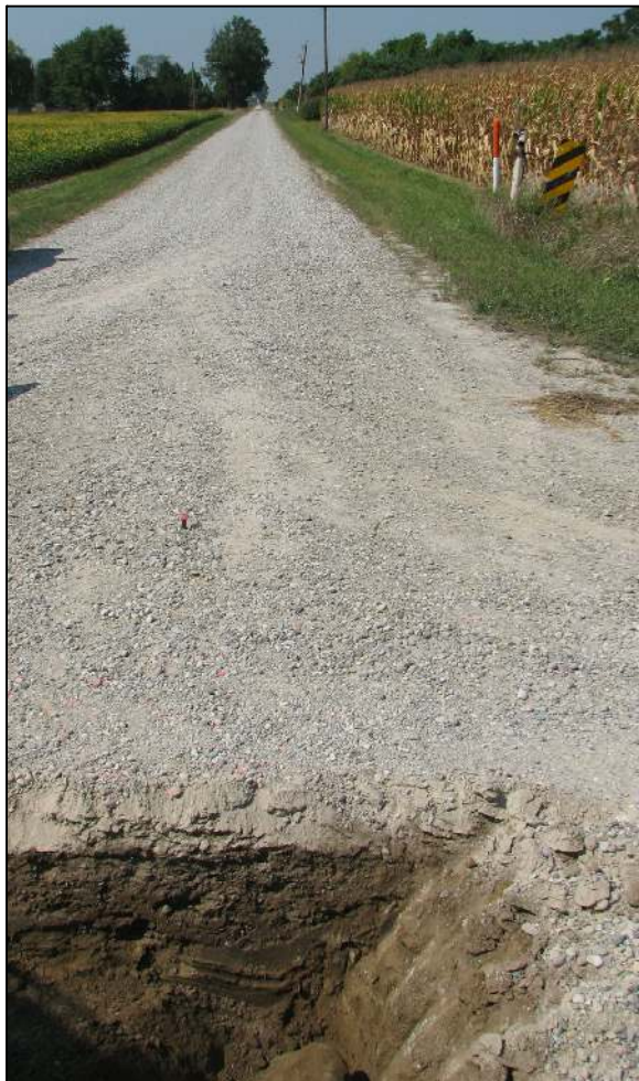
View from the east, looking across the stone and west along County Road 900 North.
