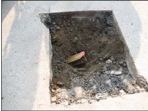
The section of leaning railroad rail, exposed with the high point painted pink.
