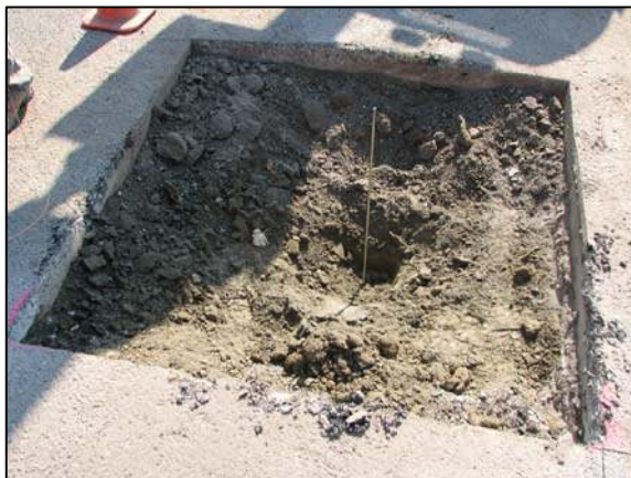
The hole in the road bed after the stone was removed.
