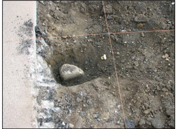
View from above and south showing the stone exposed and the position of the rebar (marked by the plumb-bob).
