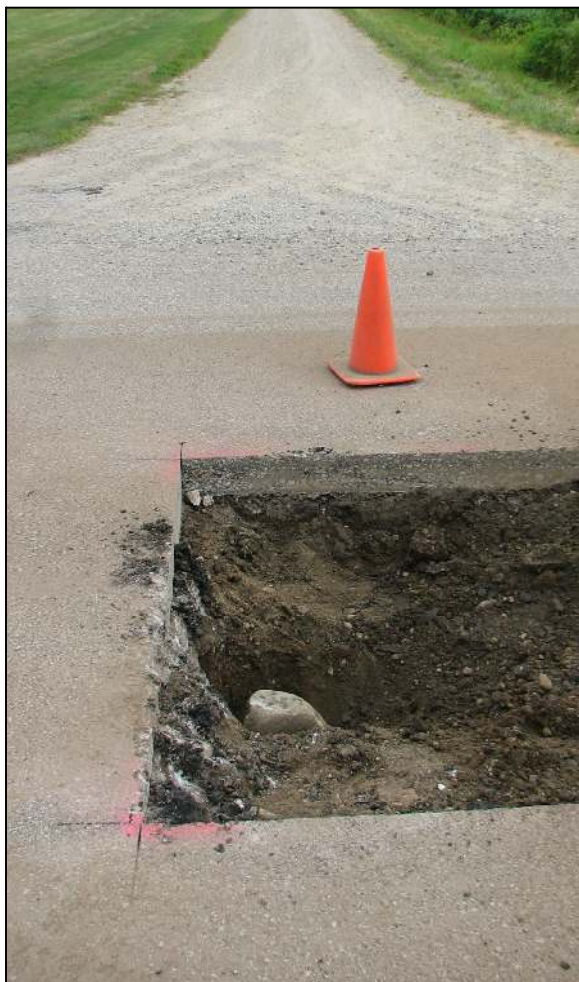
View from the south, looking across the stone and north along County Road 700 East.
