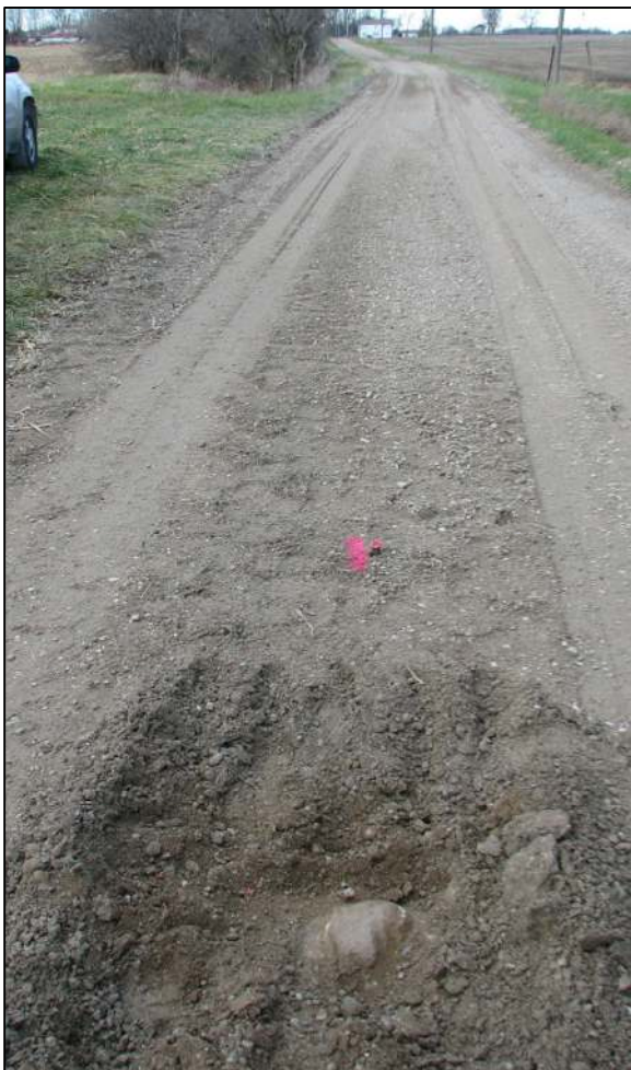
View from the south looking across the stone and rebar and north along County Road 900 East.
