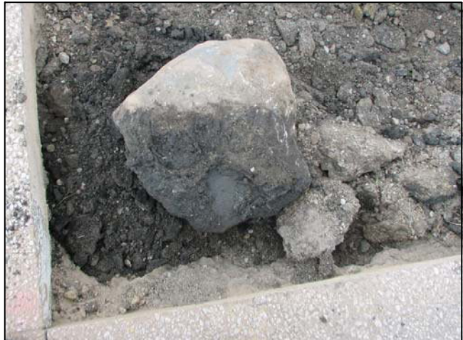
Corner stone removed from ground, showing extent to which stone was embedded in clay. Approximately 10" of stone was in clay and 7" protruding into bottom of road bed.
