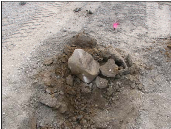
View of the stone displaced from the road bed.
