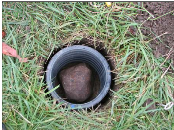
The stone at corner one prior to being encased in concrete with a Harrison monument set above.
