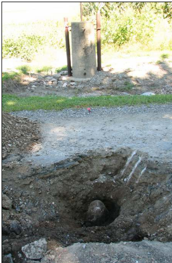
View of the stone and the large concrete post on the north side of the road.
